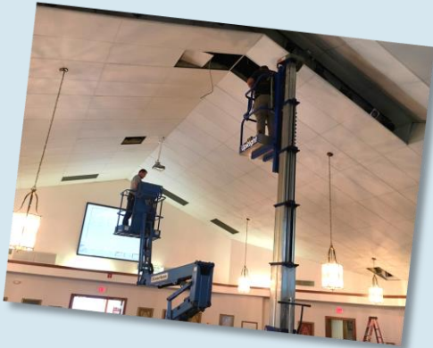
Both lifts extended and work on projector and spot light in progress
